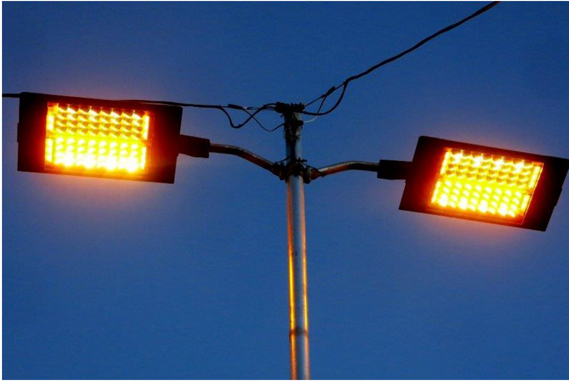
An amber LED fixture test installation on the NAU campus.
